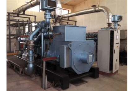
Gas-fired Generator – Working Mine, Pingdingshan, China
