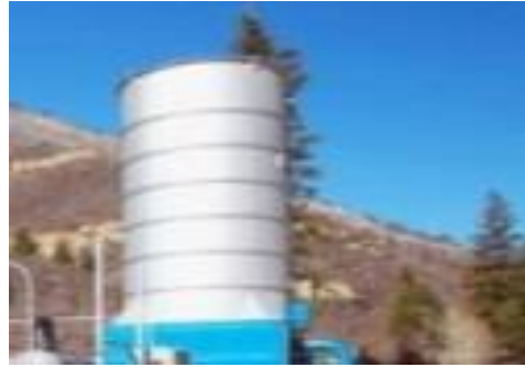
Abandoned Mine Methane Flare Colorado, USA
