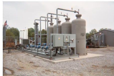
Gas Conditioning & Upgrading System for Gas Pipeline Sales Abandoned Mine, Illinois, USA
