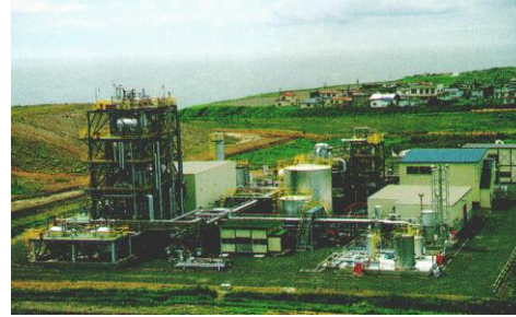
Methanol Production Plant
