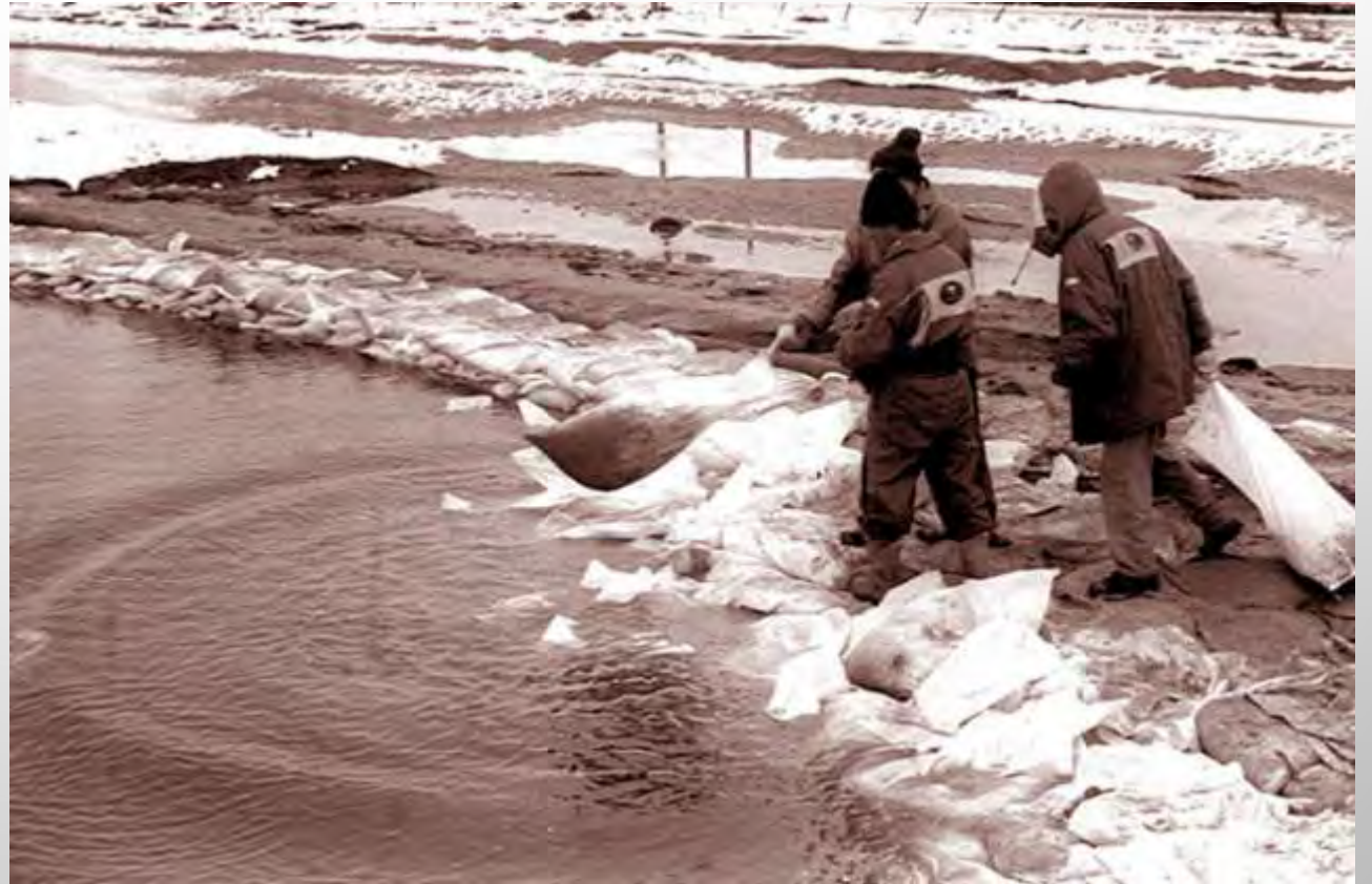
Figure 5. Workers trying to block the breach with sandbags (source: Ecomagazin.ro)
