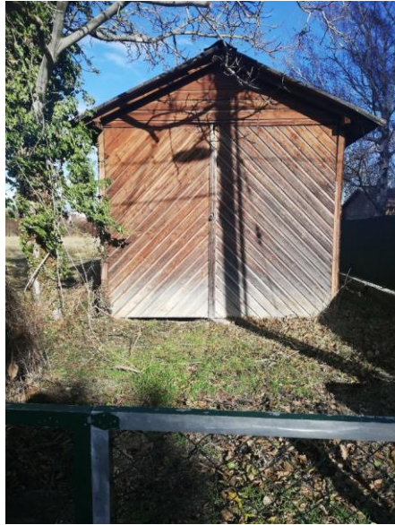
Picture II from local inspections
