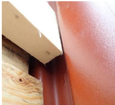
Figure 7.72 Beam too short
