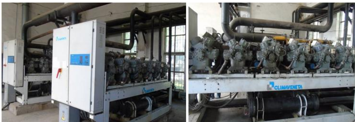
Figure 8. General view of an obsolete chiller running on R22
