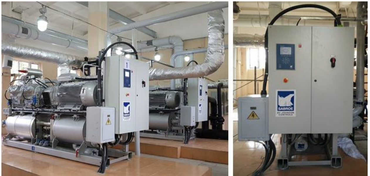
Figure 9. General view of the new chiller running on R717.
