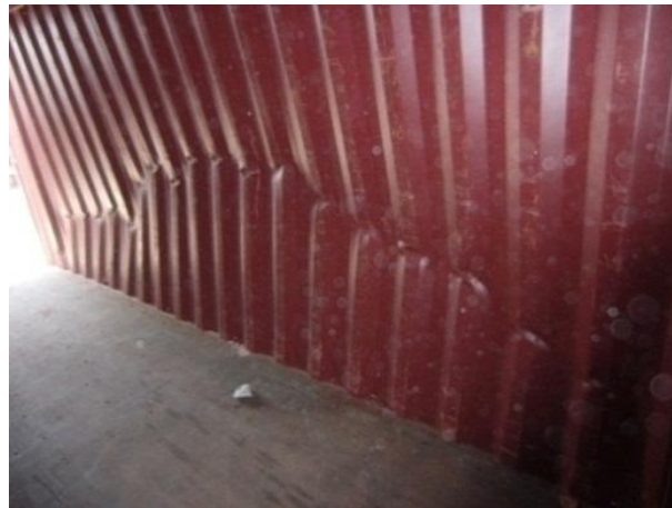
Figure 7.50 Damaged CTU side wall
