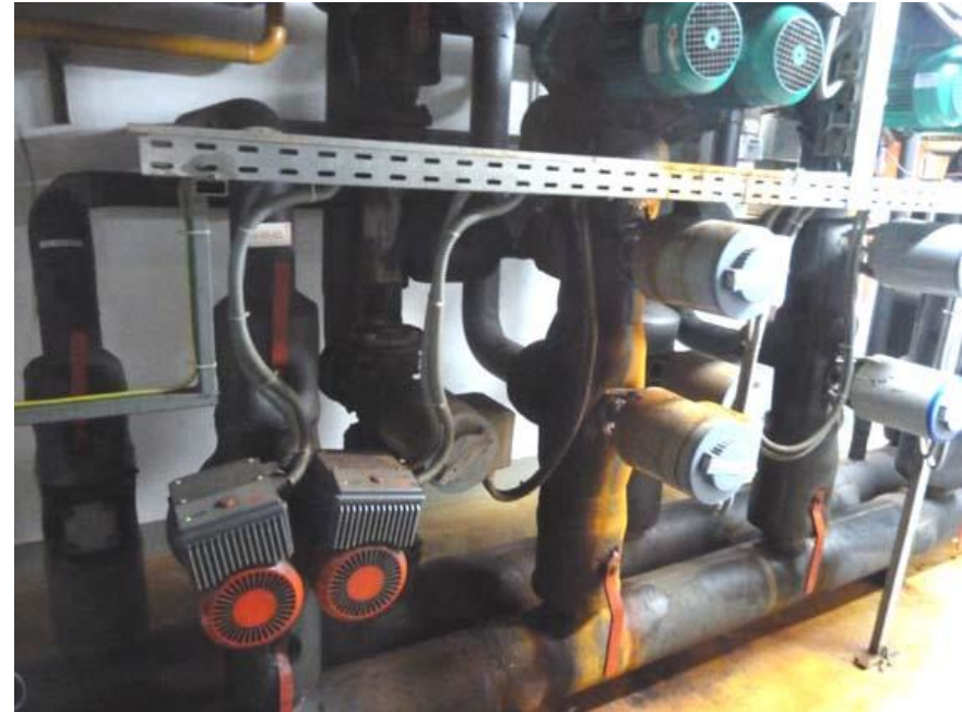
Main COLD water distributor with 3 cooling circuits
