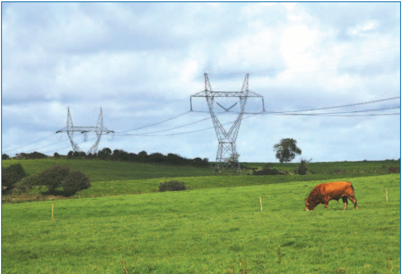
Figure 2: Photograph of a 400kV Single Circuit Intermediate Tower
