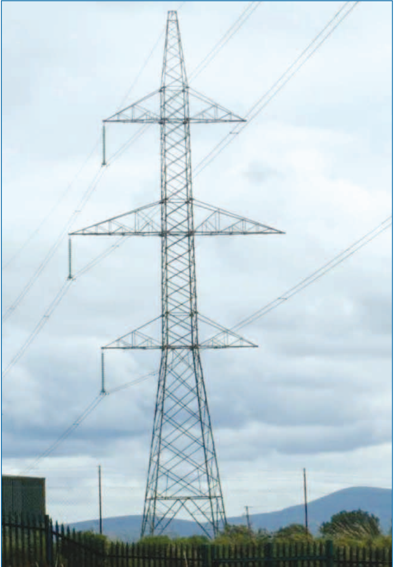
Figure 3: Photograph of a 400kV Double Circuit Intermediate Tower
