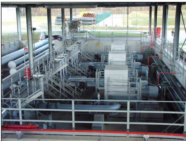
booster pump station
