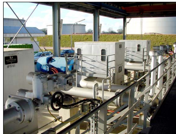
main pump station
