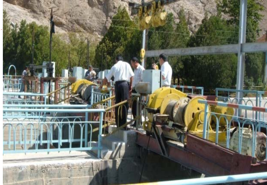
Isfara Headwork: Automated systems (2013) © Natalia Alexeeva
