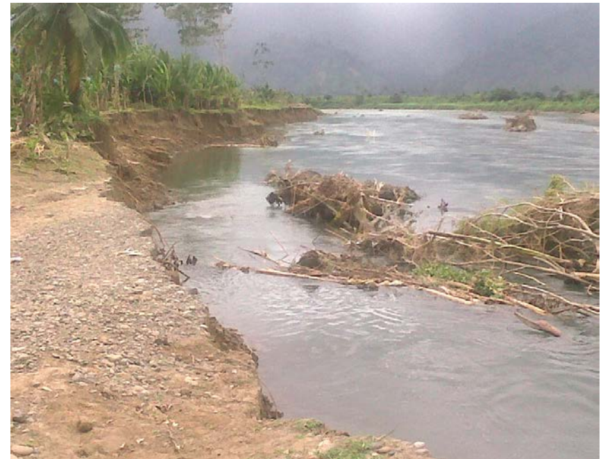
Destroyed road by changes in the river path. To the left, plantain crops ( Costa Rica )
