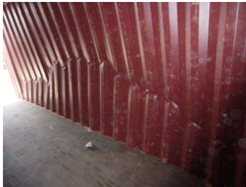
Figure 10-39 : Damaged CTU side wall
