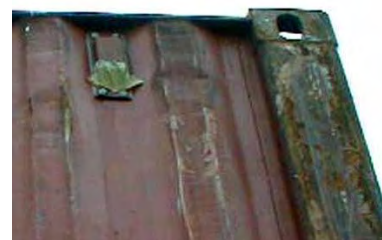
Figure XII-12 : Vent tapped over
