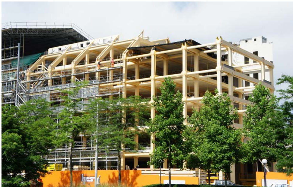
Fig. 1 Timber frame of the new Tamedia office building with clearly visible timber joints (Image source: Thomas Rohner, St. Gallen/LIGNUM)
