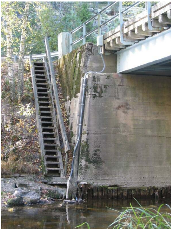
Figure 5. The hydrological measurement station.
