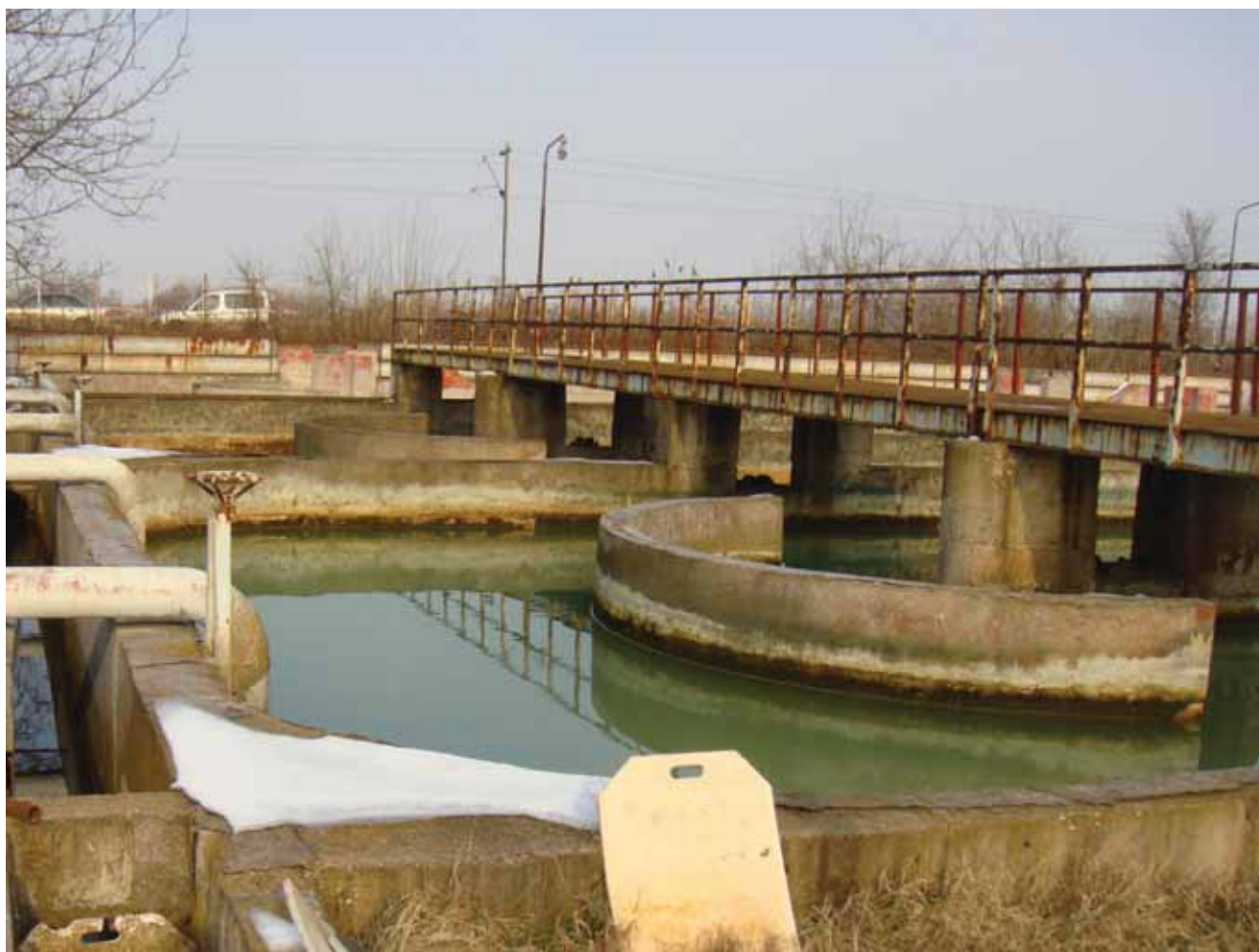
Photo 6.1: OHIS waste water treatment plant
