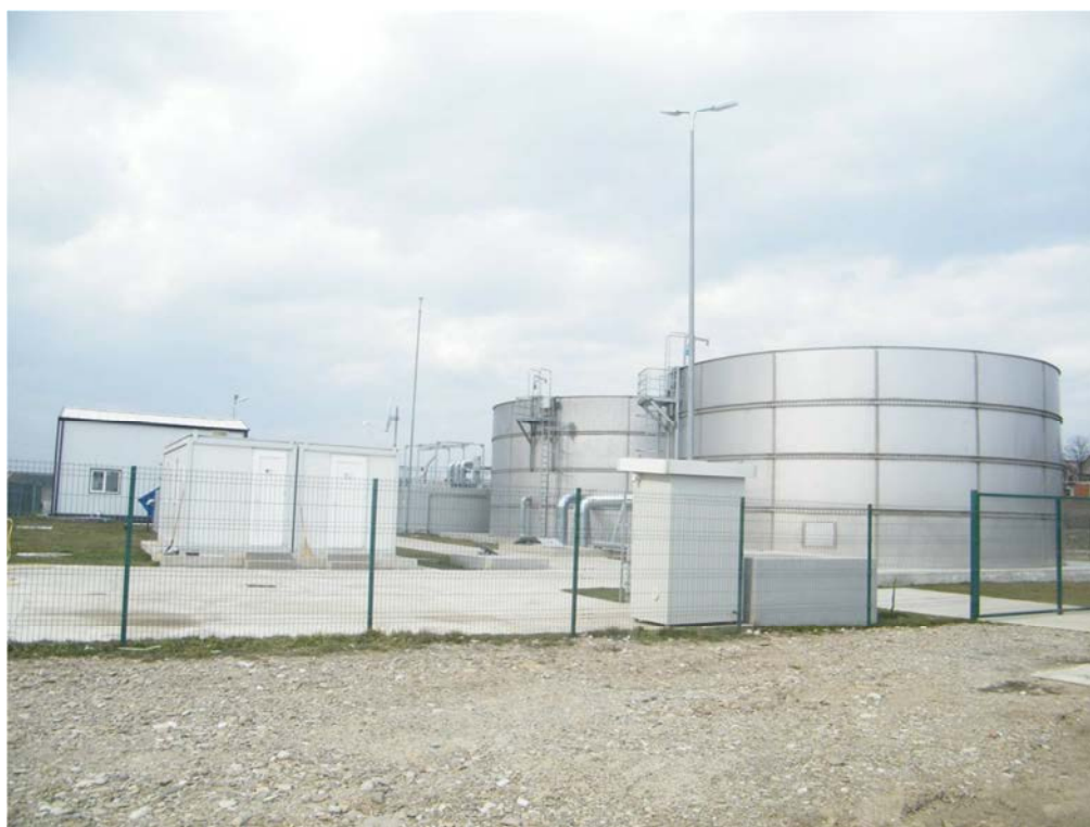
Photo 7.1: Maracineni wastewater treatment plant
