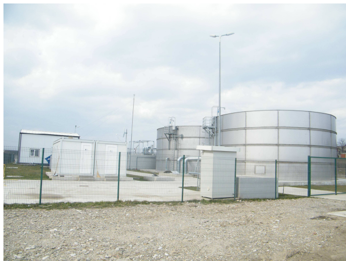
Maracineni wastewater treatment plant © Mr. Constantin Dumitru
