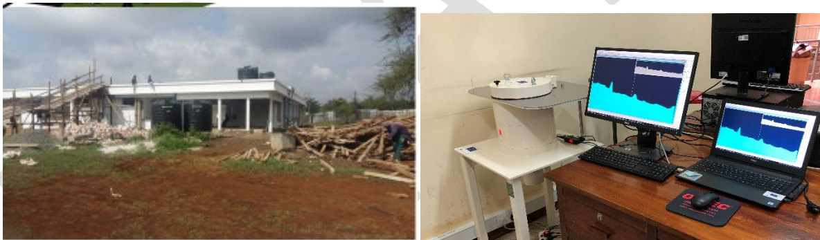
Figure 18. Infrastructure and capabilities – new facilities in advanced construction with new equipment at Tanzania Atomic Energy Commission (TAEC) Arusha, August 2018
